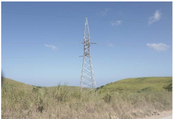
Plate 6 - 132 kV Transmission Line Towers 28m high
