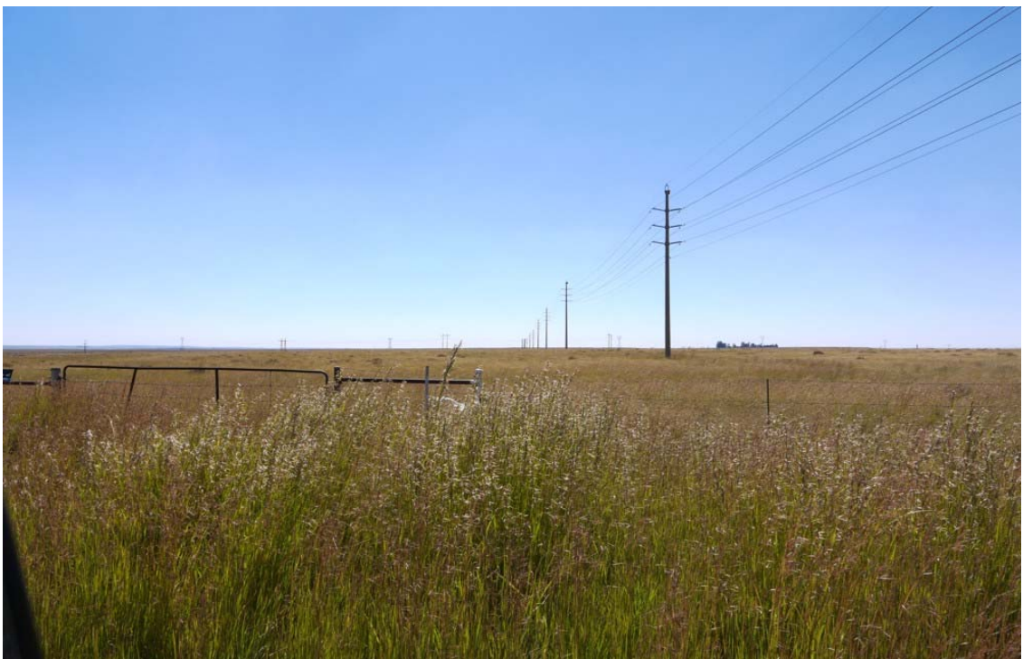
Plate 12 - A view along the line of a monopole 132kV overhead power line. Note towers on the horizon approximately 2.5km away are just visible.
