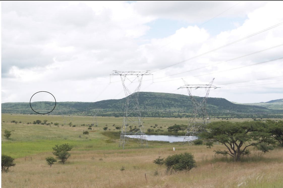
Plate 9 - Existing 400kV overhead transmission lines. Clearance of the servitude is the most obvious landscape change at a distance (approximately 5-7km)
