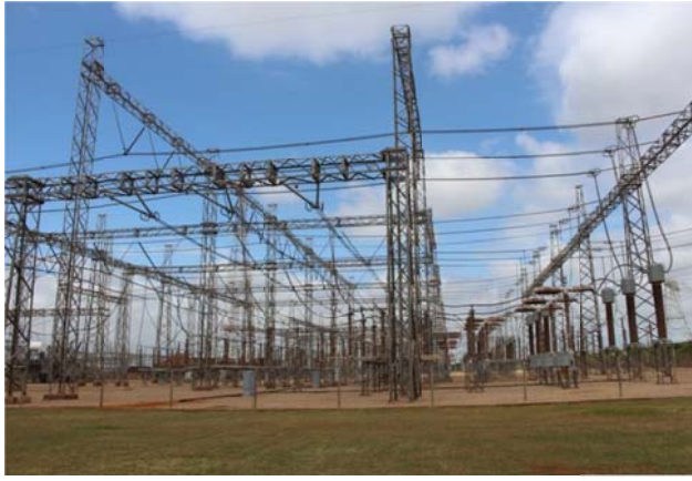
Plate 1 - Sub-station Busbars maximum height 22.5m
