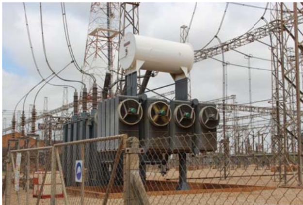
Plate 3 - Transformer showing oil reservoir and fans for cooling
