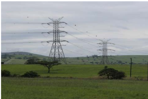
Plate 5 - 400 kV Double Circuit Transmission Line Towers 36m high
