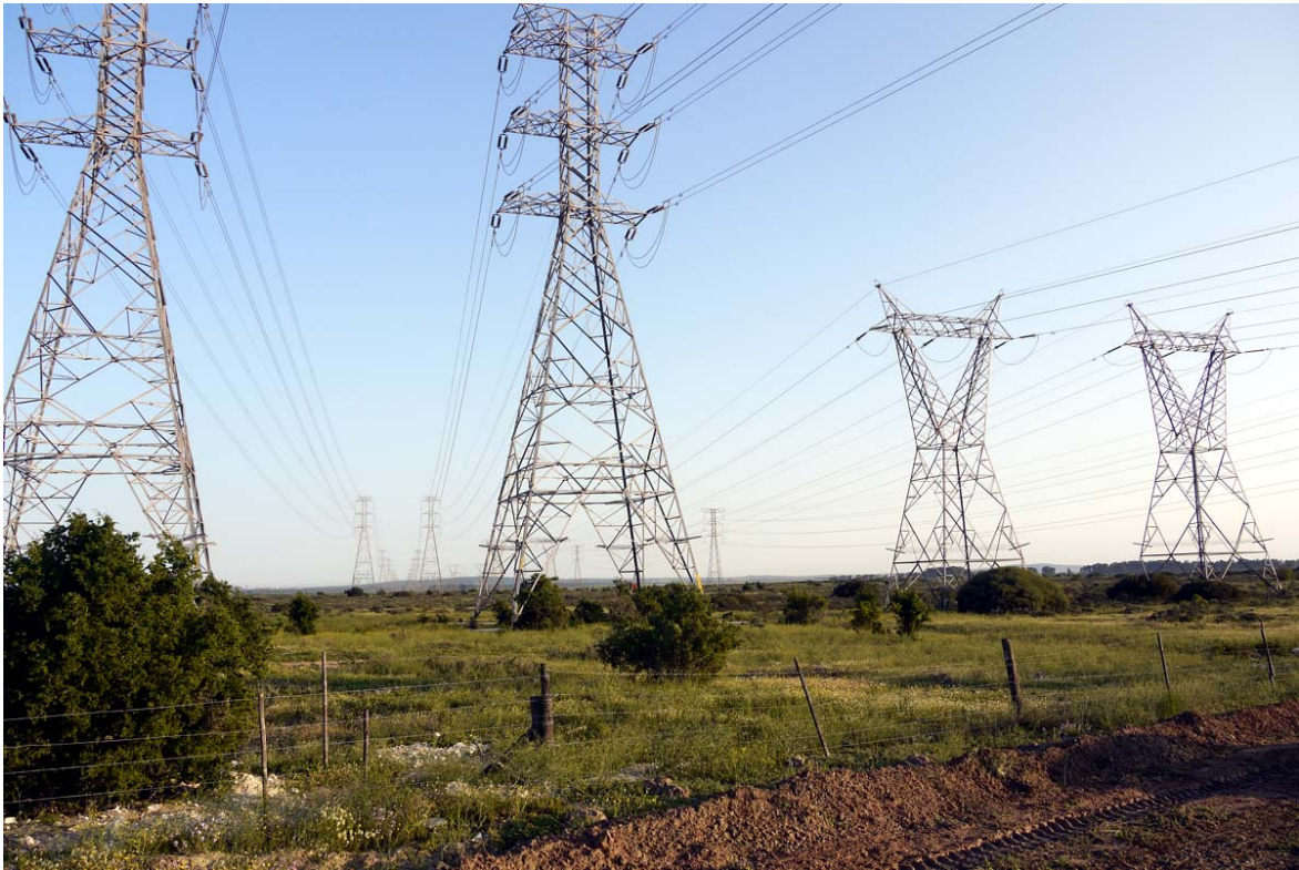
Plate 15, Viewpoint 3 - A view looking along the existing power line servitudes to the north towards TX Substation Alternative A from close to the R27 road crossing. Proposed power line alternative 3 will run close to and parallel with these existing power lines.
